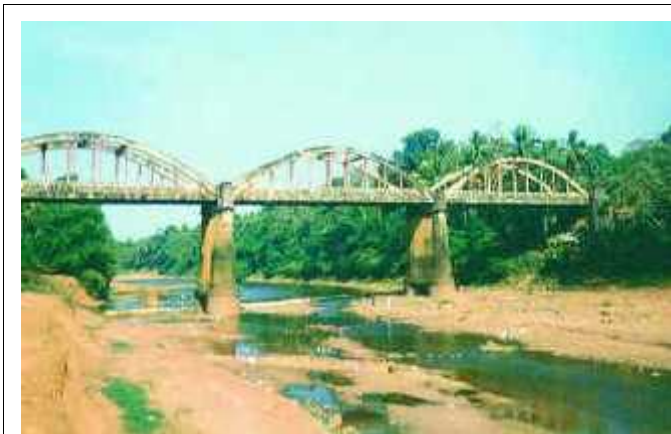
Fig 2: Indiscriminate sand mining has exposed the foundations of the bridge
