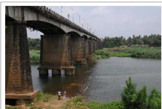
Figure 4: Exposed bridge foundation due to unrestricted mining activities
