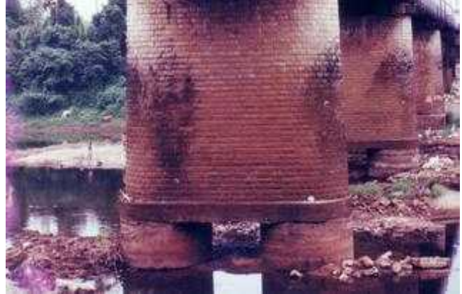
Fig 1 : Bared well-foundations of a bridge facing threat of collapse
